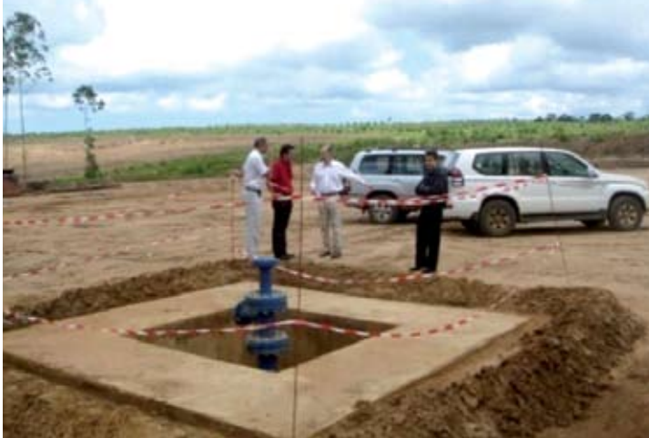
Finished production well that will feed potash-rich brine to the Kouilou production facility.
